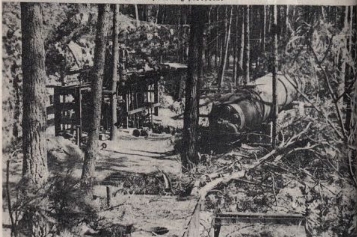
Figure 5 - The high pressure separator and control manifold of one of three dispersed plants built with equipment from Scholven is shown here. The well-camouflaged bunker on the left was the control room; manifold valve handles were extended into this bunker.
